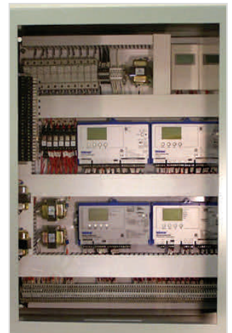
Prefabricated Control Panel
